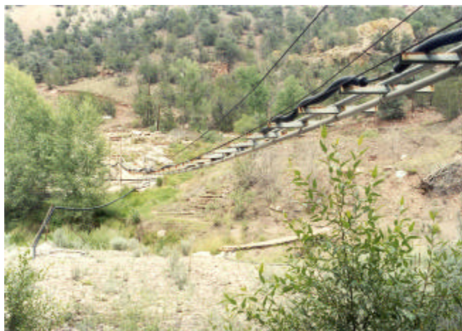
Photo 5. The suspended pipeline across the West Fork of the Gila River.
