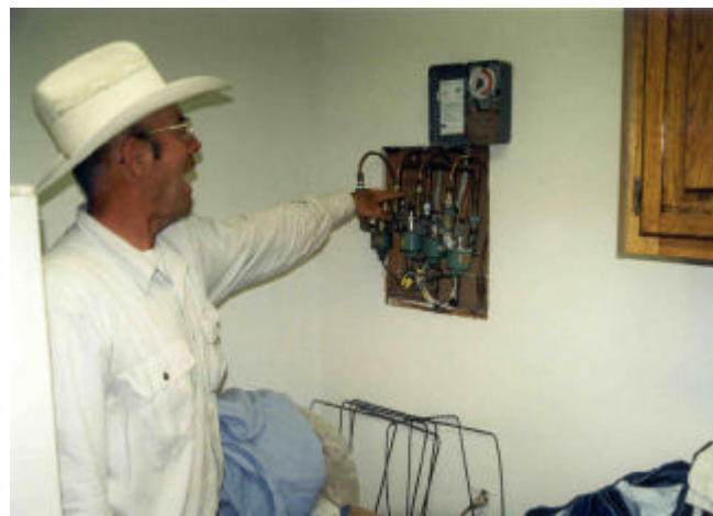
Photo 6. Allen Campbell's controls for his home heating system.
