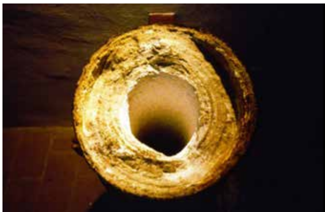
Figure 5. Scaling in geothermal pipeline (Bloomquist, 2006).
