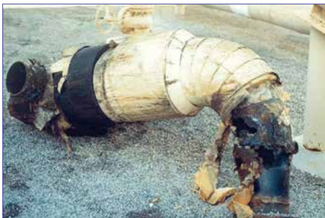
Figure 8. Corroded Steam Vent (Kagel, 2008).
