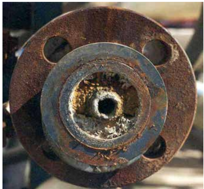
Figure 6. Corrosion of tubes (Kagel, 2008).
