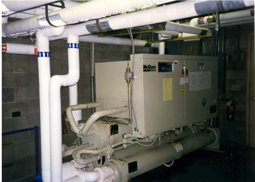
Figure 3. Photograph of one of the water-to-water heat pumps at the Inn of the Seventh Mountain.
