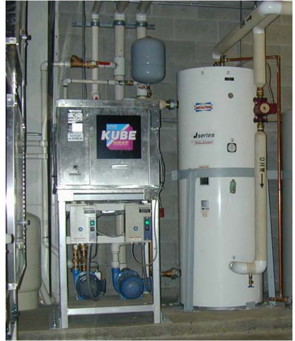
Figure 5. A 10-ton water-to-water heat pump draws heat from the earth loop to produce service hot water (showers and ice flooding) at 120°F (50°C)
