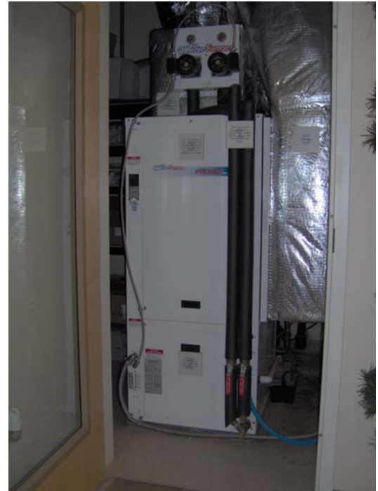
Figure 3. Photograph of a 6-ton, water-air, vertical heat pump and flow center.
