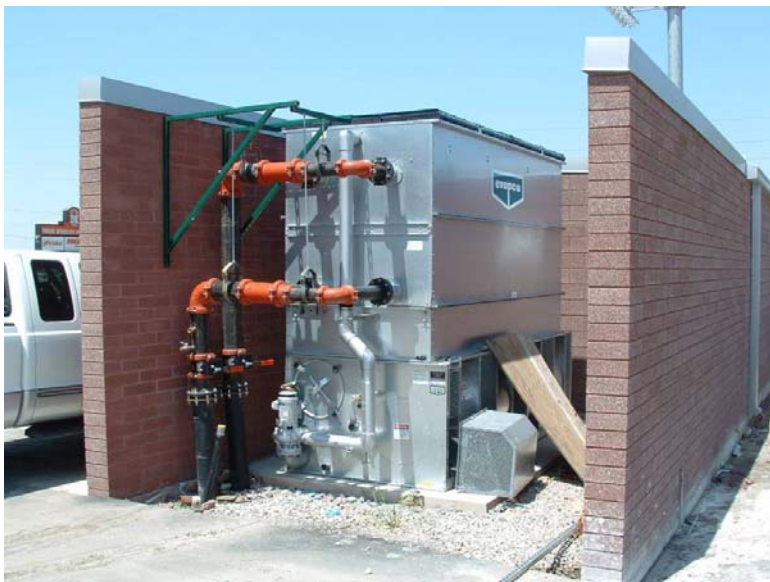
Figure 2. Photograph of the fluid cooler at the Murray High School.
